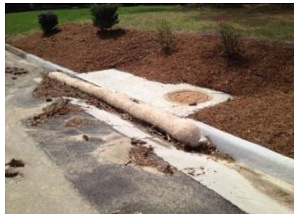
A-12: Curb Inlet Filter
